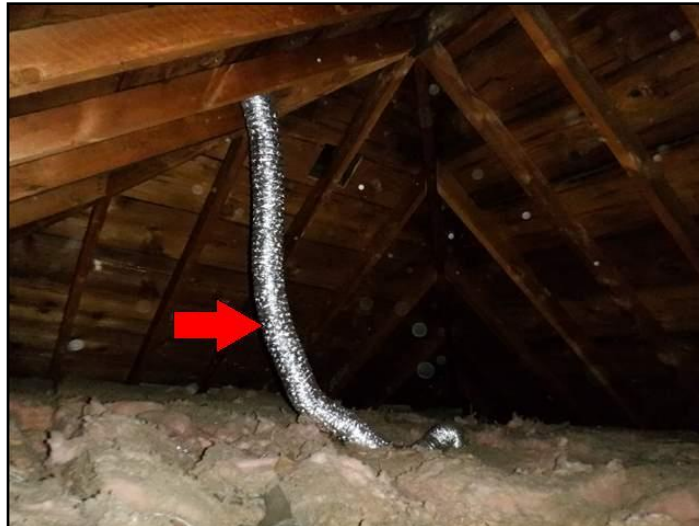
Not insulated in unconditioned space
