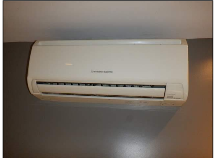
Ductless (Mini split) system
