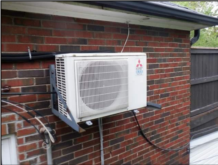
Ductless (Mini split) system
